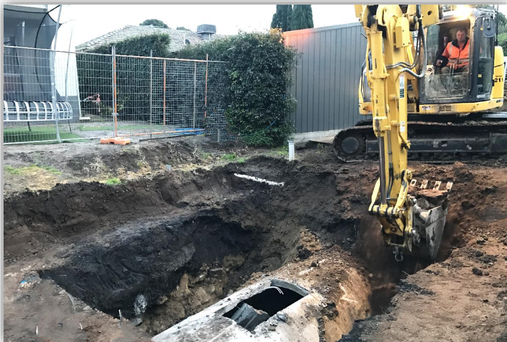
Construction of 2.5m x 2.5m Melbourne Water Pit in close proximity to residential properties
